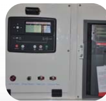
Control Panel & MCB
